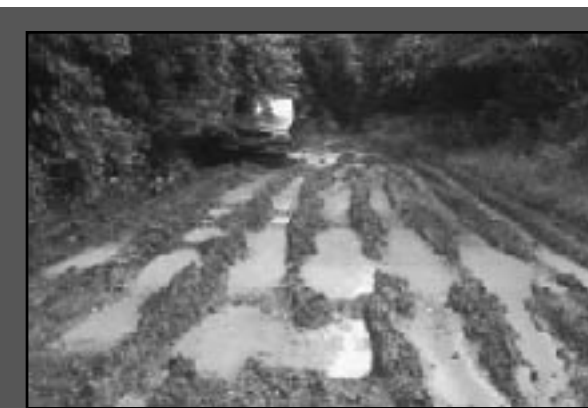
Photo A1 Avoid construction and other road activities during wet periods when possible. Alternatively, add drainage and surface stabilization to the roadway in weak soil areas for all-weather use.
